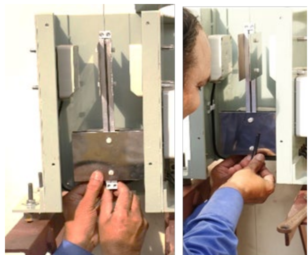
Picture 14 – fixing the plumb wire clamp at the bottom of reflector assembly
